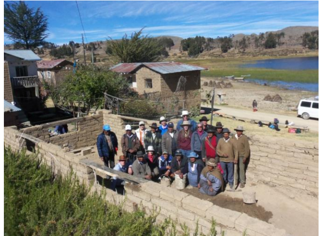
Team Onalaska with local church folks inside new Sicuani greenhouse walls they constructed during their mission trip.
